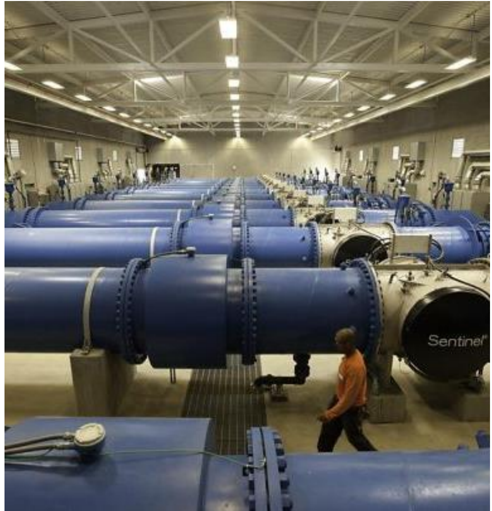
These UV reactors are part of the San Francisco Public Utilities Commission's new Tesla Water Treatment Facility. It can treat 315 mgd.
