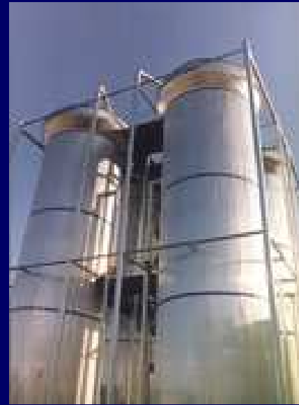
Anaerobic bioreactors (wastewater treatment)
