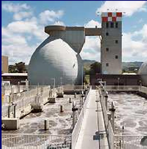
Anaerobic sludge digesters
